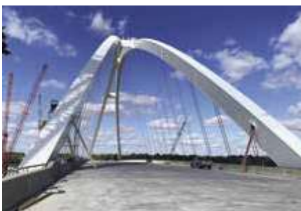
Hyper-durable FEVE resin used for the I-74 Mississippi River bridge is impervious to degradation caused by UV radiation, moisture and salt.
