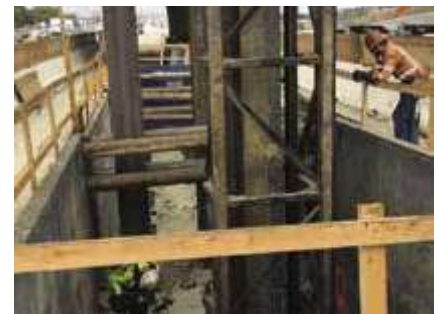
H-piles from Nucor Skyline will be used for bridge foundations on the I-405 project.
